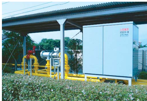
Part of city gas facilities at the Atsugi Operation Base
